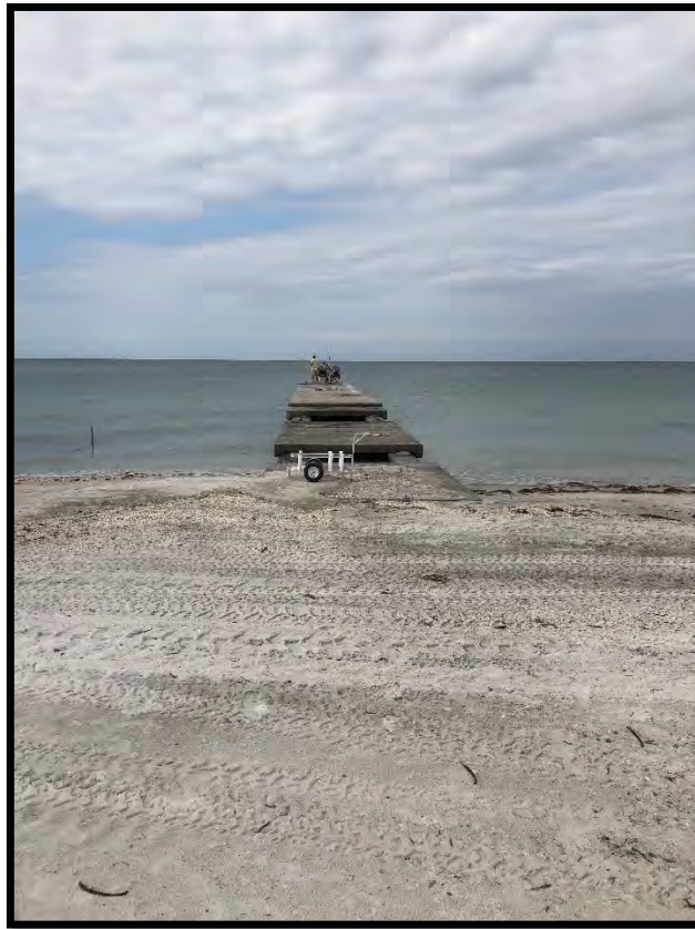
Photograph 1. Groin Facing West
