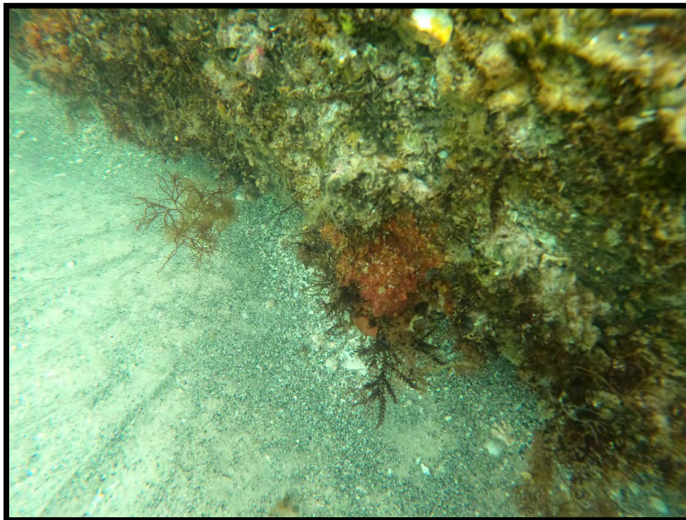
Photograph 14. Encrusting Sponge and Algae on Groin Structure
