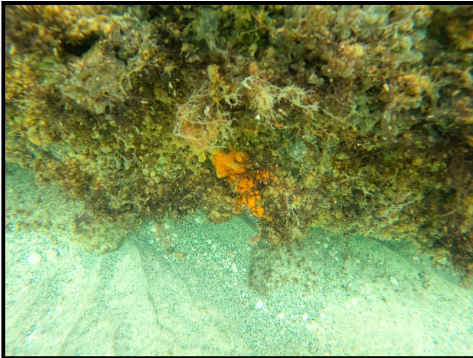
Photograph 17. Orange Encrusting Sponge and Algae on Groin
