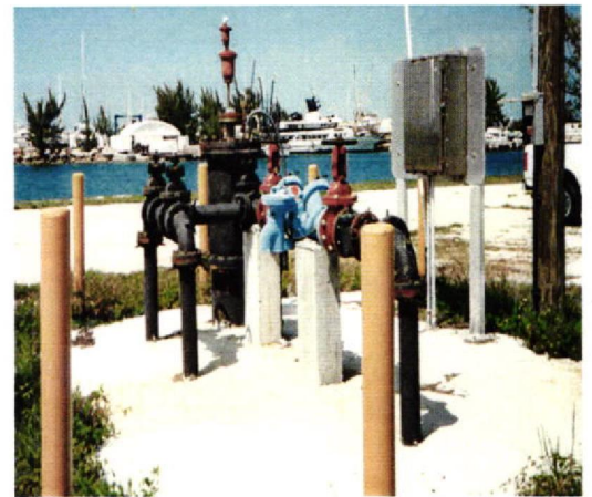
Deep Well Injection Well Head
