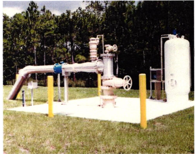
Deep Well Injection Well Head
