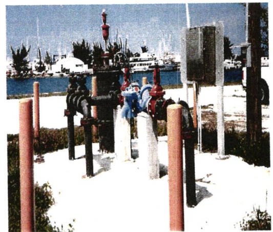
Deep Well Injection Well Head
