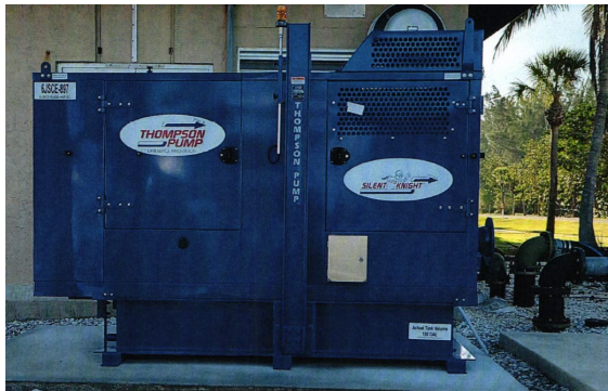
Lift Station “E” By-Pass Pump
