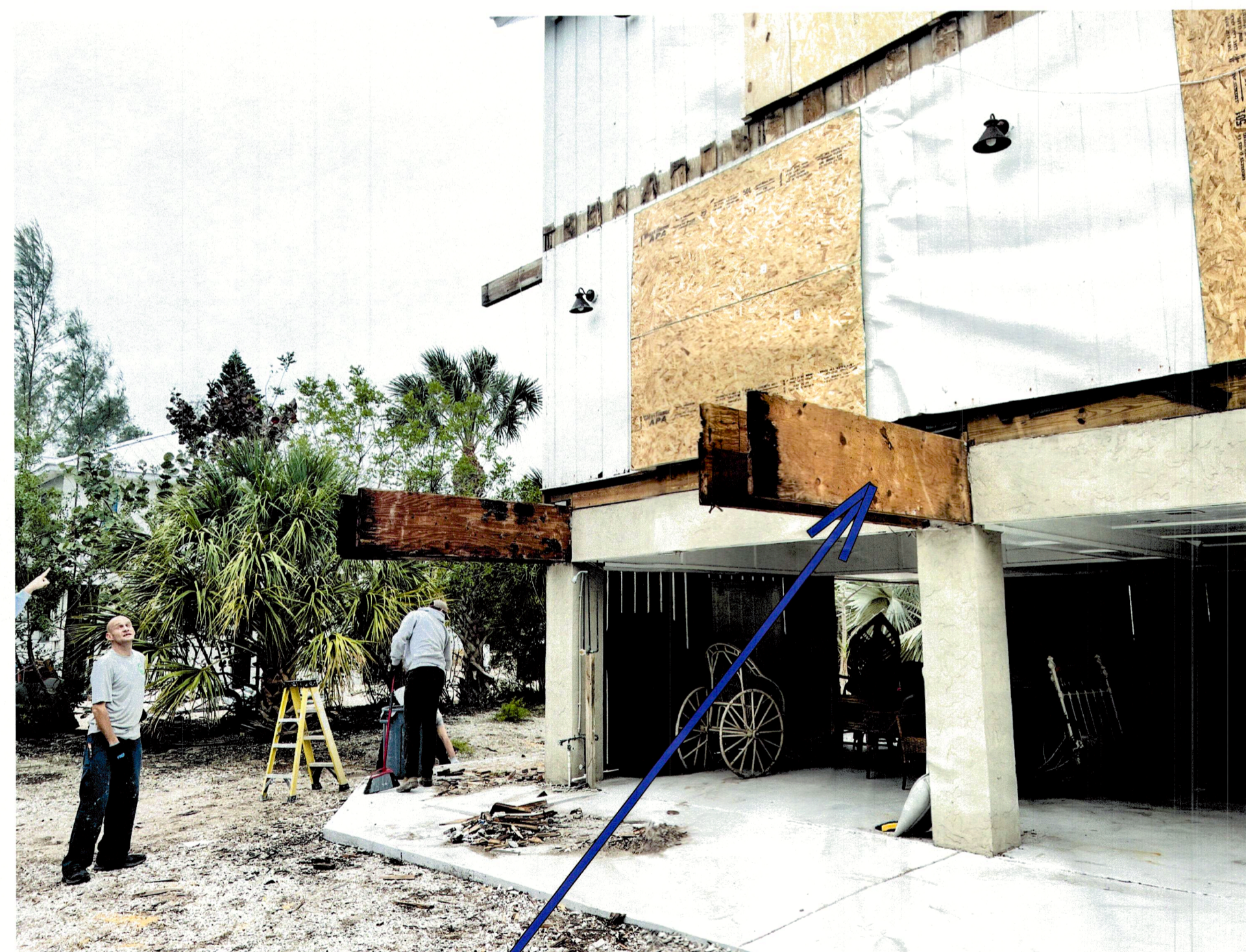
LVL cantilevers to be cut flush with house, wrapped and finished with plywood and stucco mortar to match existing
