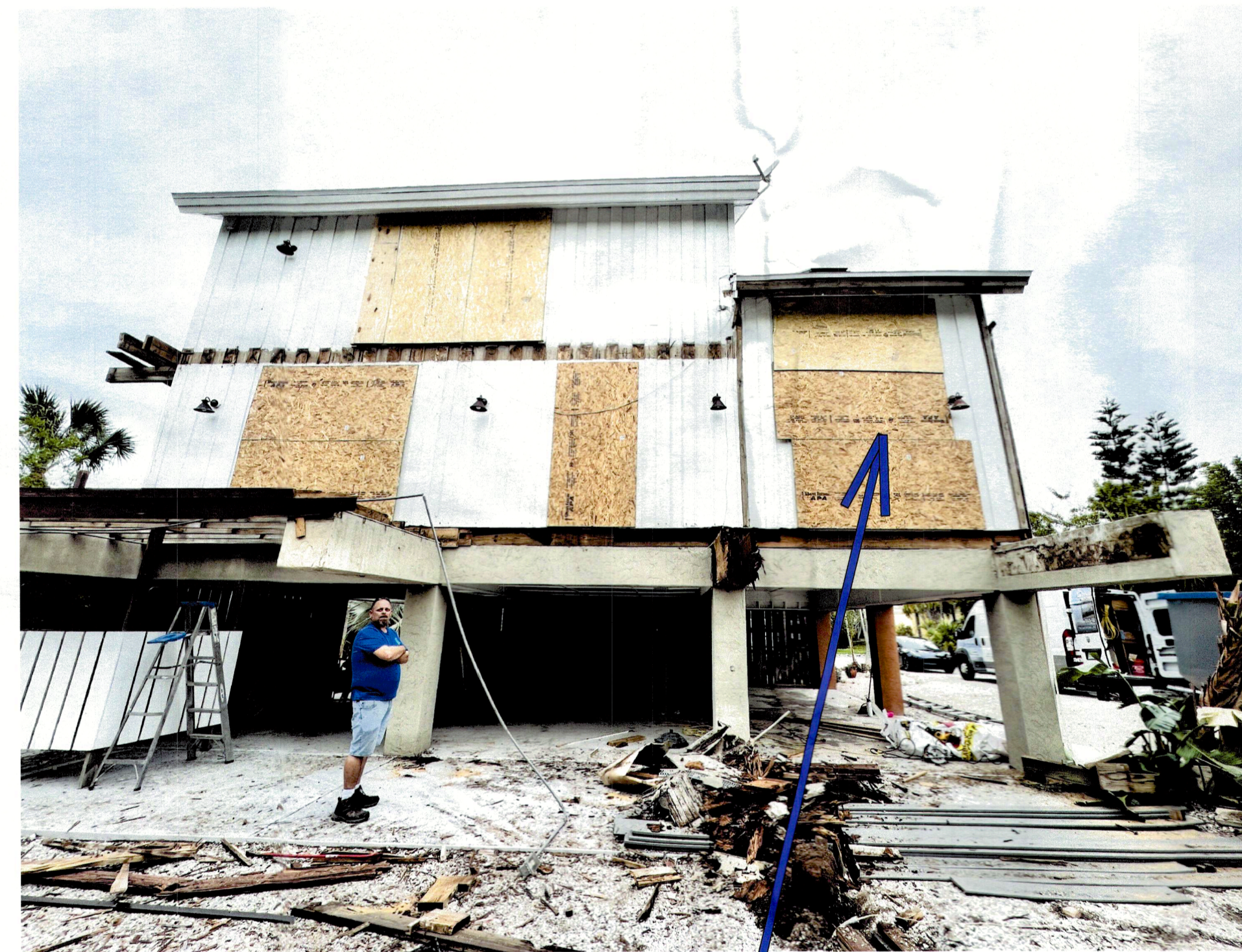
This was an existing door into the main home. The door will be removed and the doorway will be finished. No other changes to existing structure or framing.
