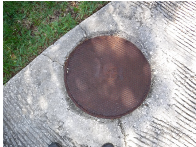
Cracks adjacent to manholes may contribute to infiltration of saltwater into utility conveyance systems in areas of regular tidal flooding.
