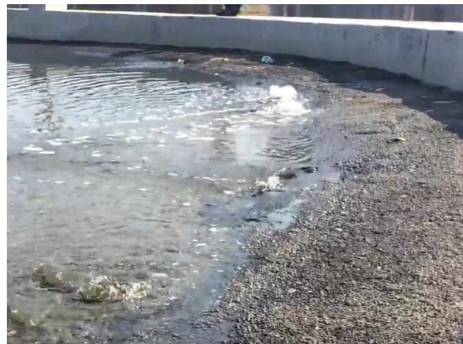
Example of road deterioration in area vulnerable to seepage during high tides (Hollywood, Florida).
