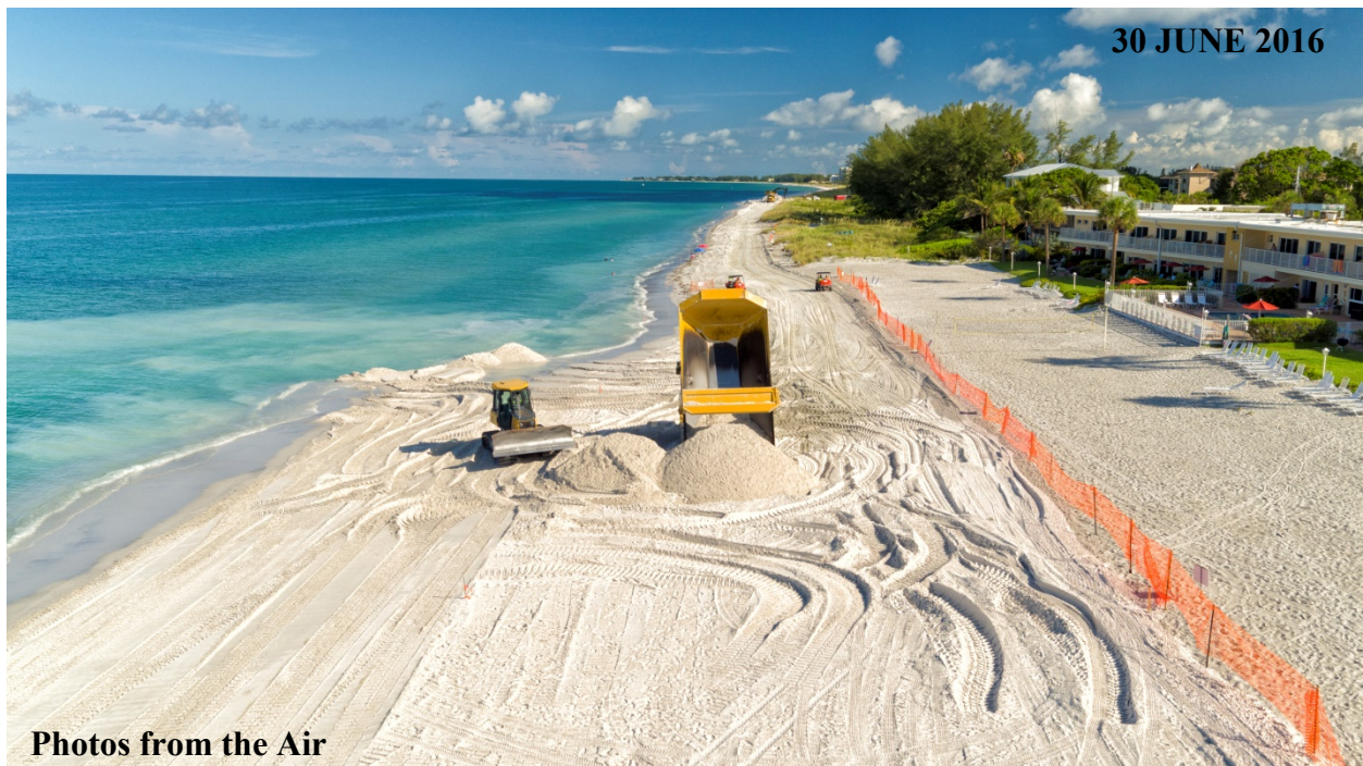
Figure 5.6 Construction operations in the vicinity of the Seahorse Resort (R-6) during the 2016 Central Key Beach Nourishment Project.
