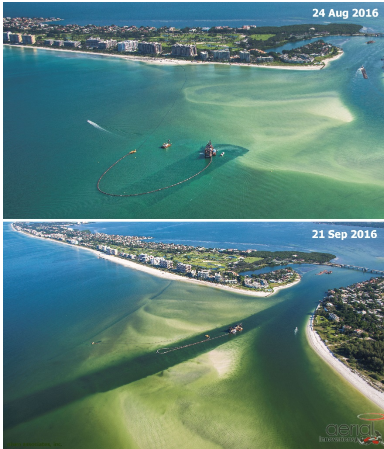
Figure EX-3 Dredge excavation of the New Pass ebb shoal channel borrow area, with sand placement to the south end of Longboat Key, (Aerial Innovations, Inc.)
