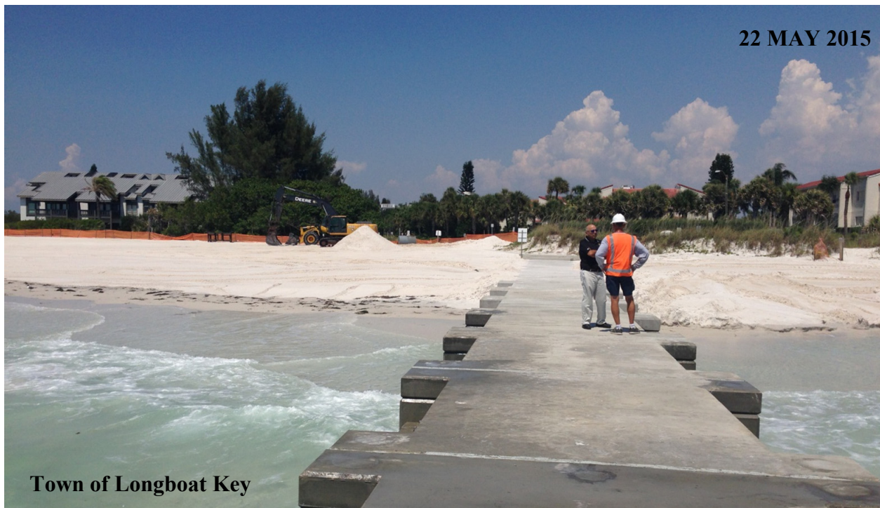
Figure 5.8 Beach fill operations following the construction of the North End Permeable Adjustable Groins at North Shore Road in Longboat Key, FL. Sand was sourced from E.R. Jahna Greenbay.
