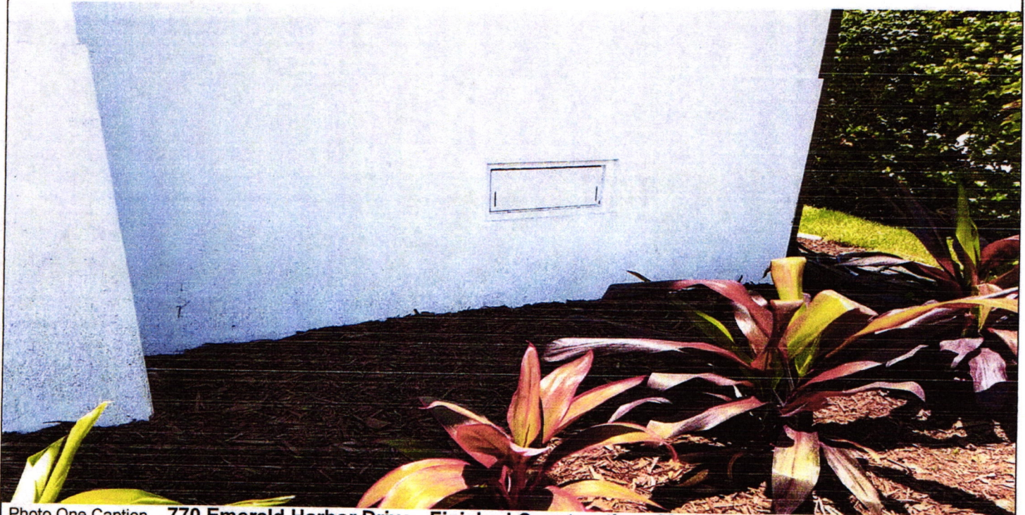
Photo One Caption 770 Emerald Harbor Drive - Finished Construction - Vent Photo June 2018
