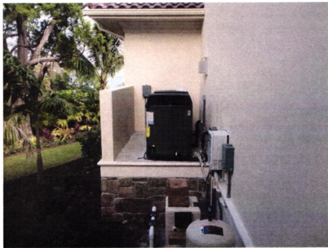
AIR CONDITINER EQUIPMENT 11/20/2015
