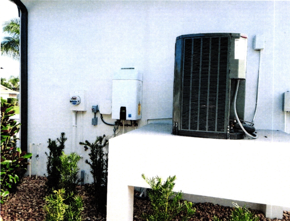
(11/21/2023) Elevated AC Platform= 9.0', Tankless Water Heater= 9.3'
