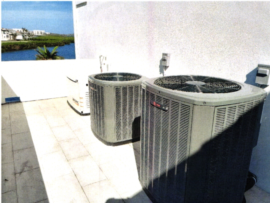
(11/14/2024) Elevated AC Units and Generator
