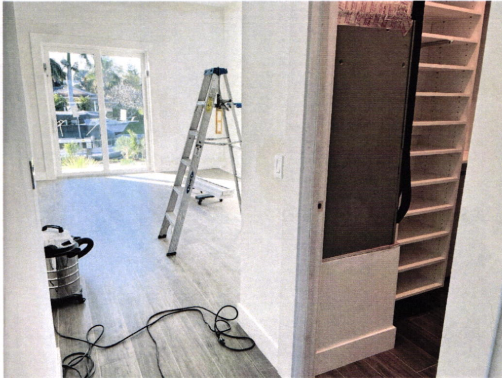
(03/29/2022) Air Handler on 1st Level Living Area
