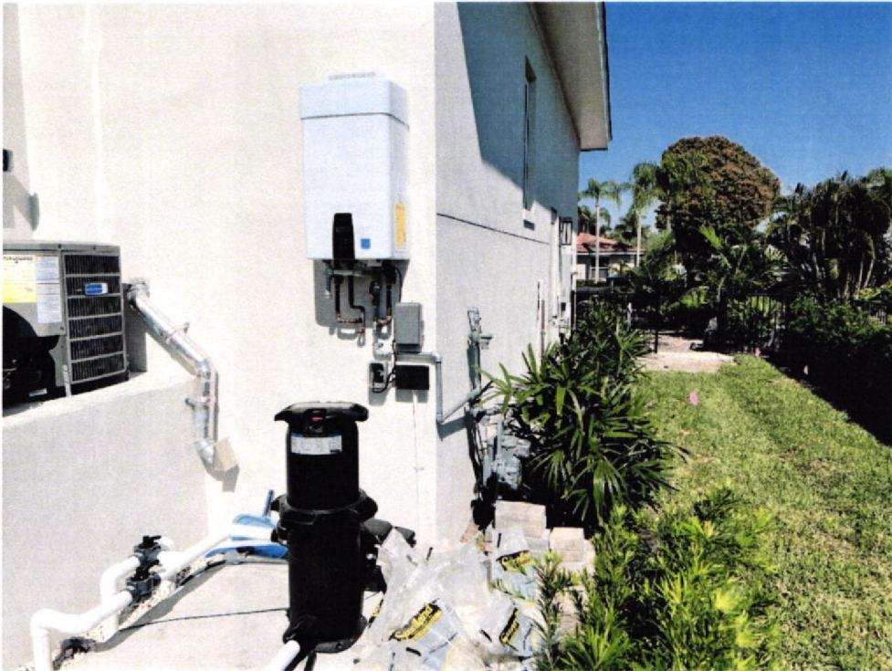
(03/29/2022) Tankless Water Heater on Left Side of House
