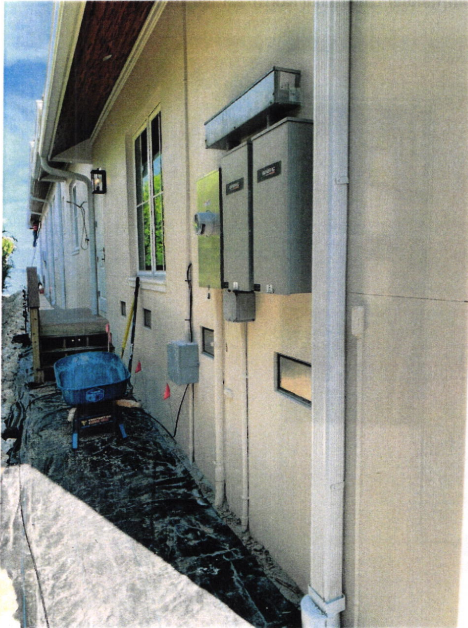
(01/26/2021) Typical Flood Vents in Garages, and Elevated Generator Panels and Electric Meter Box on North Side of House
