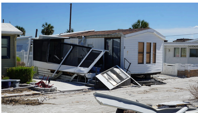
A severely damaged home in the Twin Shores community on Longboat Key after Hurricane Milton (Carter Weinhofer-the Observer).
