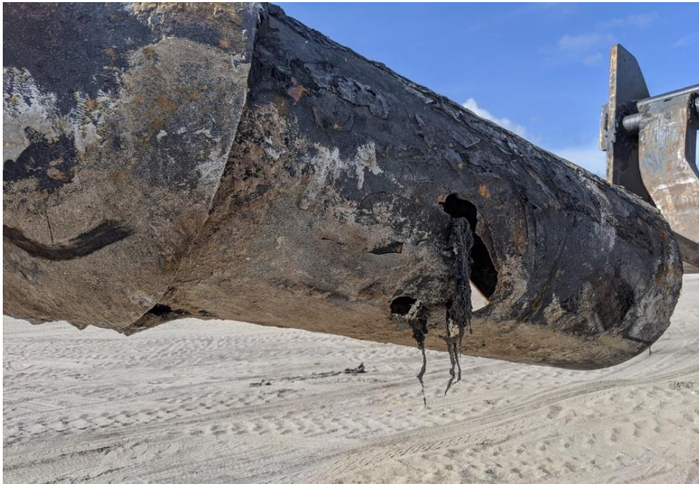
Figure 1-1 Photograph of Existing Force Main Leak
